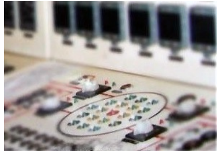
Type 09I Reactor Plant Control Panel
